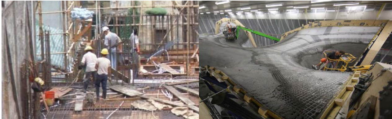
Fig. 1: Current typical concrete construction and innovative construction method by Block Research Group
